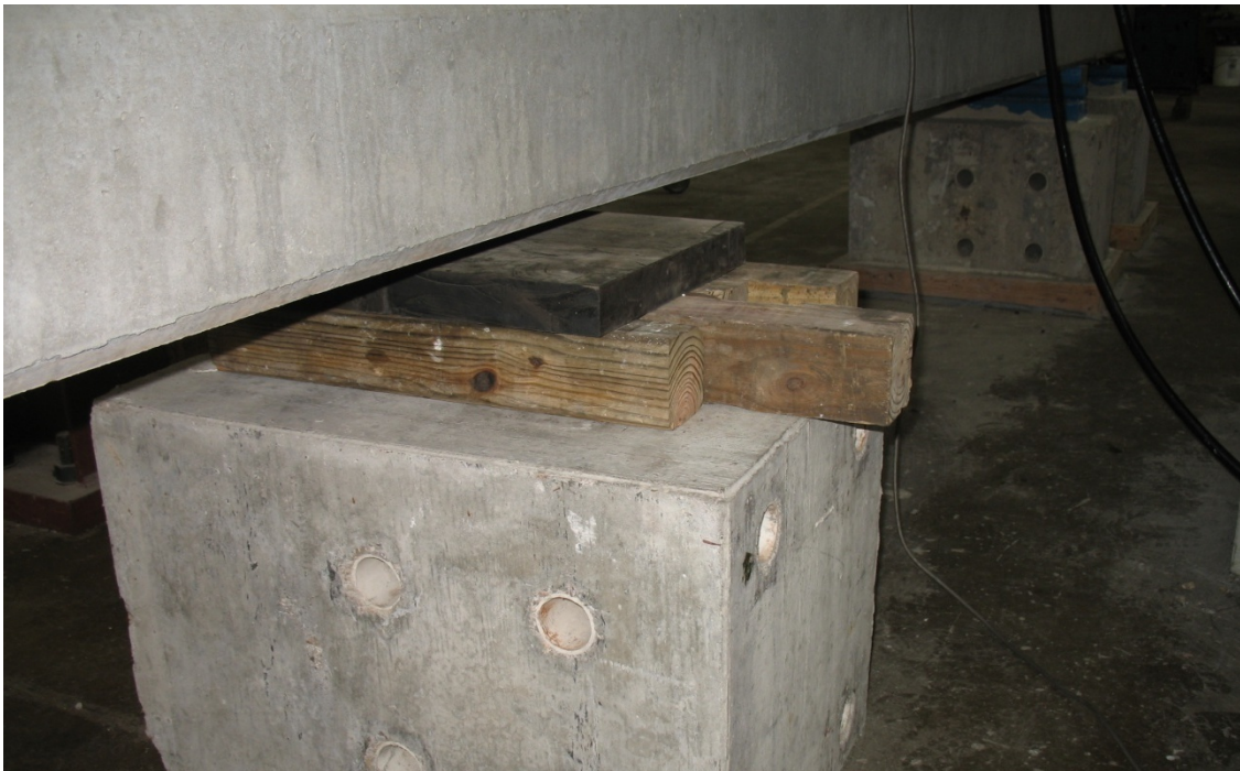
Figure 5.11 Stopper Block used to Catch Beam after Failure
