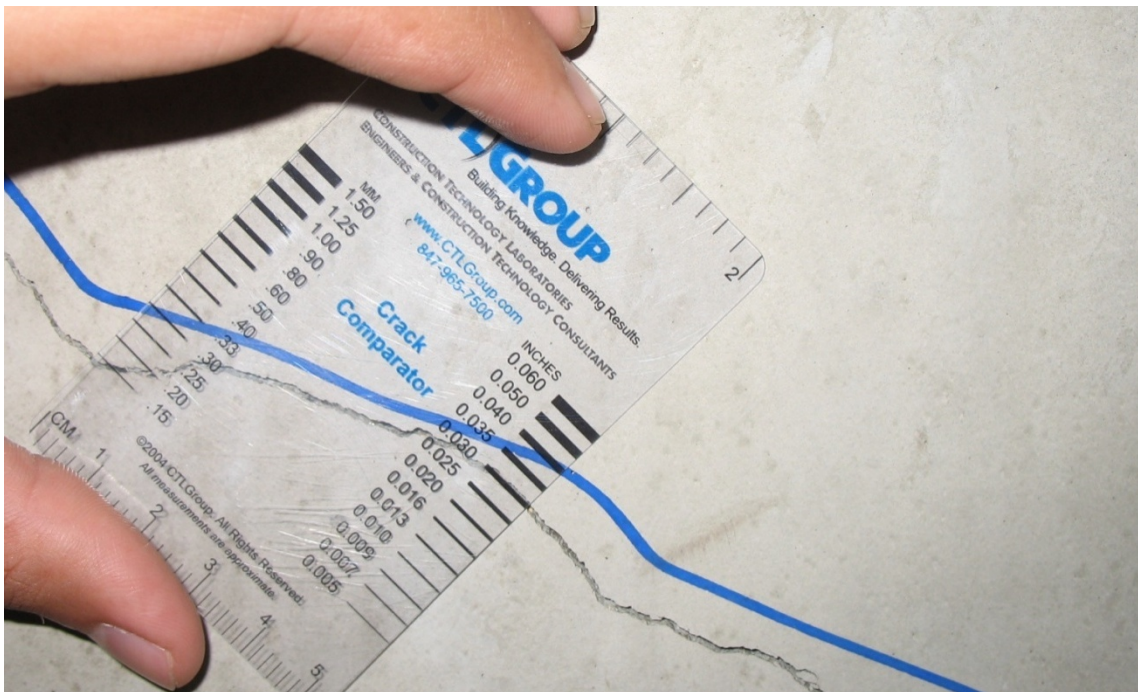
Figure 4.9 Measurement of Diagonal Crack Width
