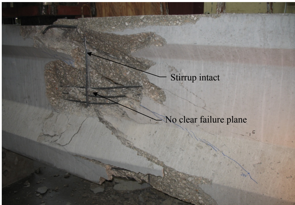
Figure 5.10 Web Crushing Failure
